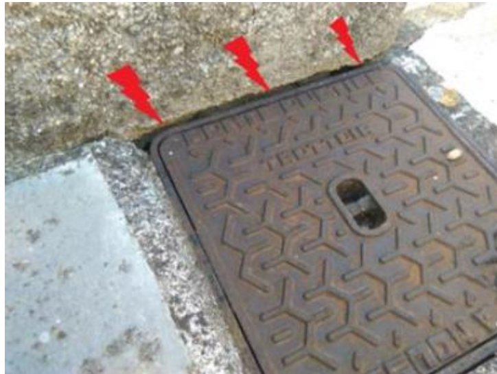
Figure 2. Plaque de regard mal scellée
